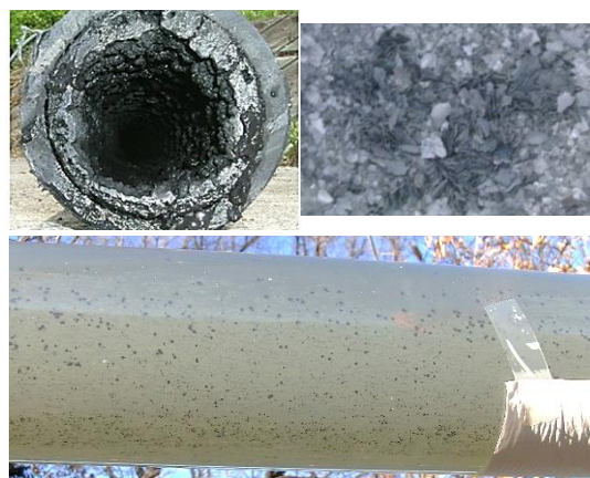
Fig. 1 (Left) The drainage pipe ( \phi=150\text{mm} ) for the leachate from the landfill site is clogged with hard scale only 5 years after the beginning of the operation. (Right) All the flakes consisting of the scale collected at the exit of the drainage pipe have the same curvature as that of the inner wall of the pipe, which shows that the solid scale nucleates on the inner wall of the pipe. (Bottom) The incipient stage of the formation of the hard scale has the appearance of small black dots attached to the inner wall of the drainage pipe.
