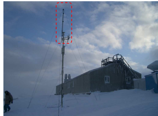
Figure 1: A low frequency radio antenna (vertical mono-pole) installed at Ny-Ålesund on Mar. 2010.
