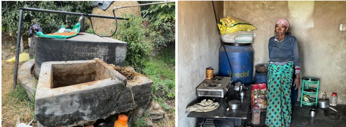
Figure 1. A view of installed biogas digester and a user of biogas for cooking in the study site
